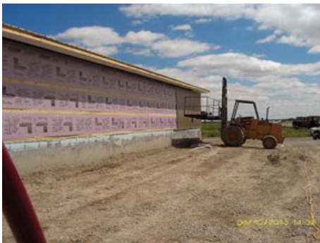
Viëga foam insulation, installed inside and between the building's girders, will help regulate temperature. Photo by Yvonne Dick
